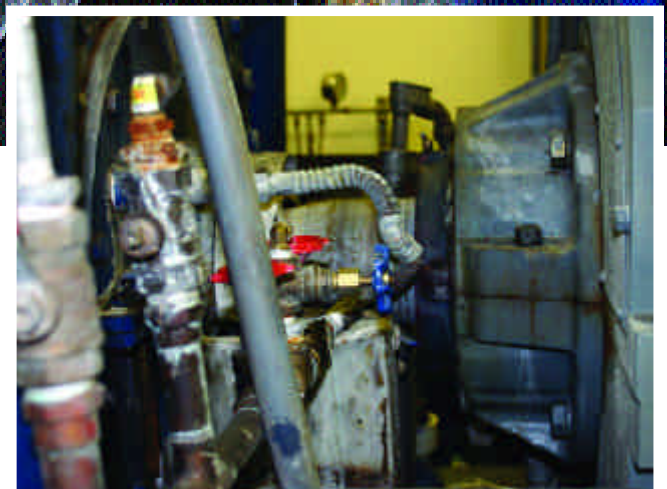
This generator is installed with a Cooper 01 BCF508EX (Expansion) bearing in a flanged housing turning at about 1200rpm.
